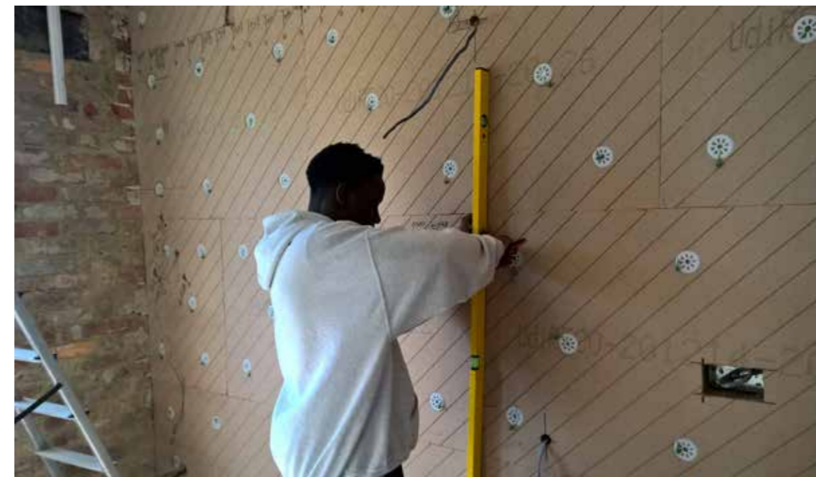
Installation of wood fibre insulation boards internally (Source: Back to Earth & ASBP)
