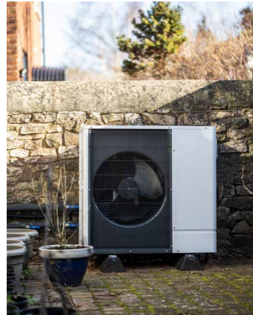
Image of an external condensing unit for an ASHP. Source: Rob Coombe
