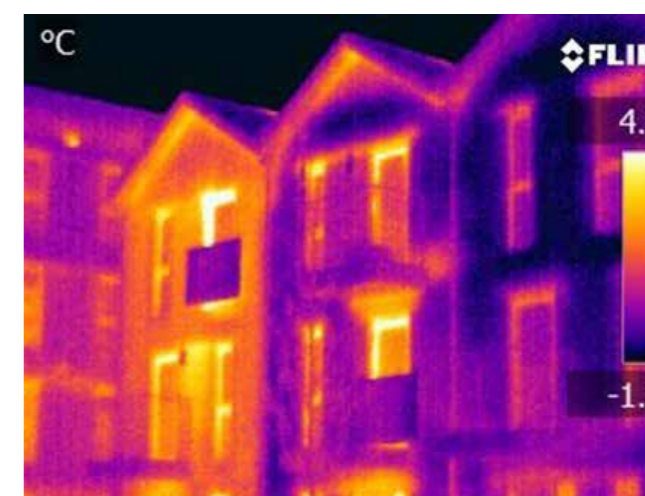
An image of the difference in heat loss between identical homes, but the end house has yet to have cavity wall insulation installed (source: Jez Wingfield, UCL Energy Institute).
